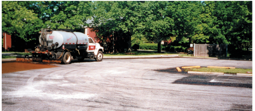
After sweeping the street, Interior Emulsions Ltd. spray applies CRF Restorative Seal. In less than an hour fine aggregate is applied, then drag-broomed to fill cracks and voids.
