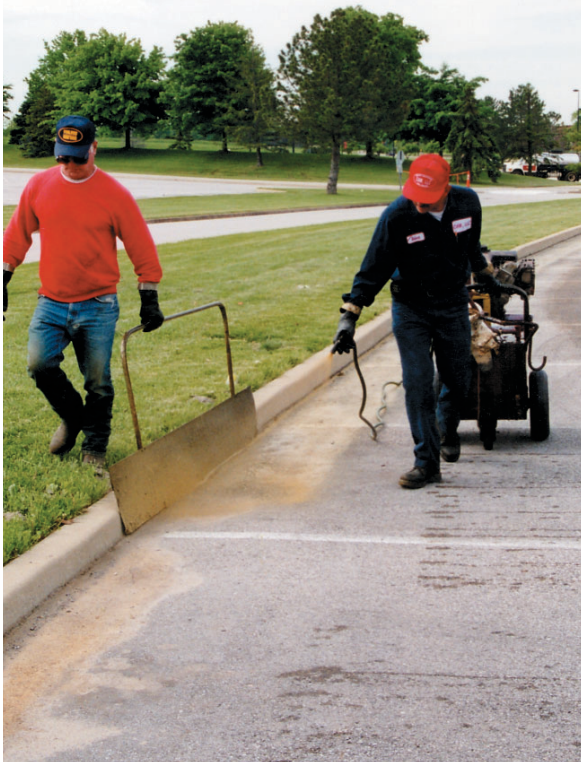
CAM LLC's Robert Brown and a laborer applying Reclamite to pavement areas not reached by the spray truck.
